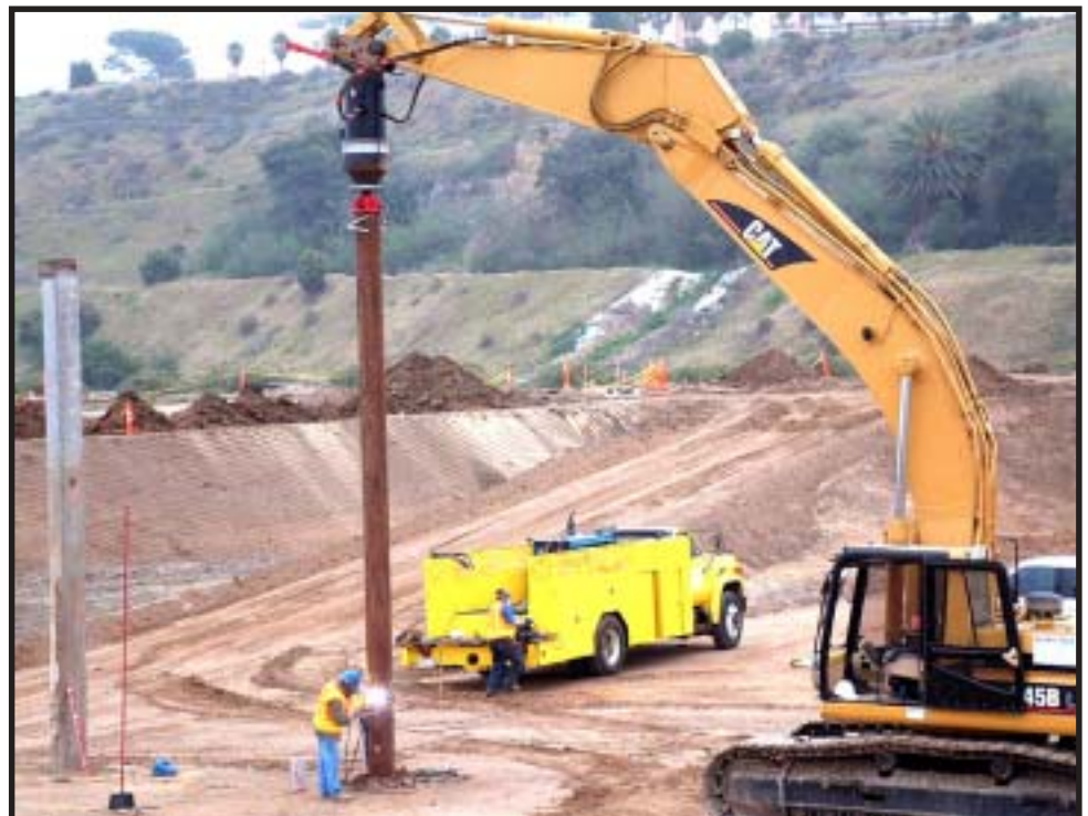
Two sections of 26 foot pipe are being welded together at the job site in the Los Angeles basin. This is the first time that concrete filled steel piers have been screwed into the ground to provide a deep foundation system.
